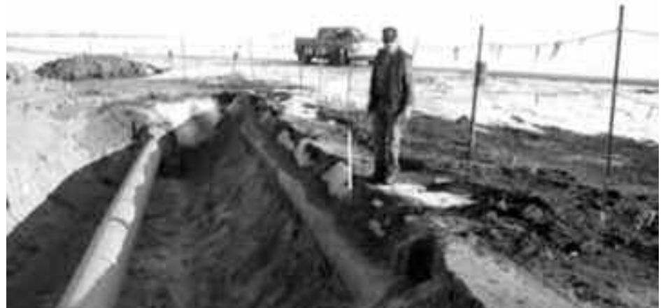
The chances are that if you do have a buried pipeline on your land, and if it has been there for any length of time, it may be a whole lot closer to the surface than you can possibly imagine.
