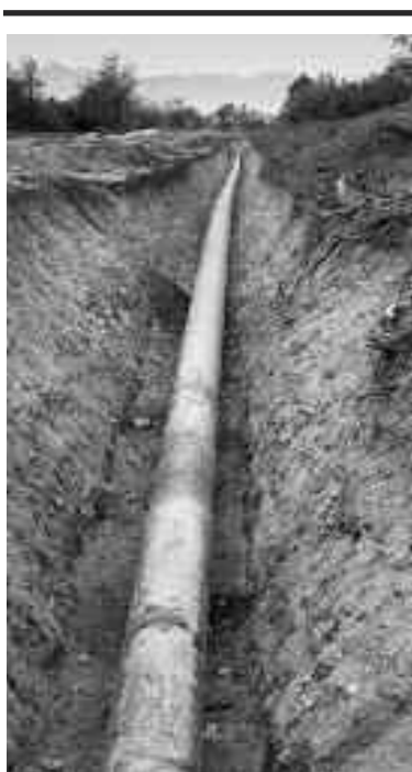
Although pipeline companies often say that they allow “normal” farm equipment and “normal” farming operations to take place over top of the pipeline, at the request of the federal regulator, they refused to define what normal or “normal weight” might mean.
